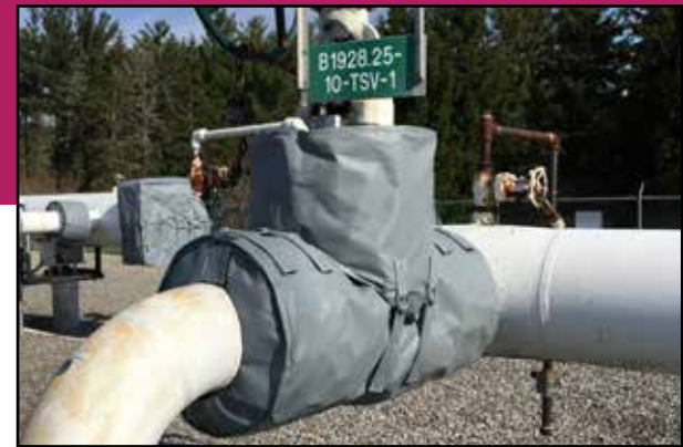
SSS-500-TAFT OIL PIPELINE - SHUT OFF VALVE
